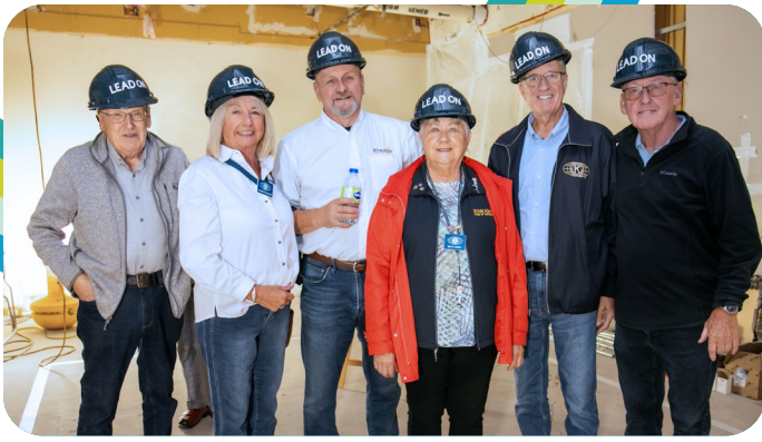
Members of the Kiwanis Club of Dartmouth joined us for a tour of the MRI Suite under construction
